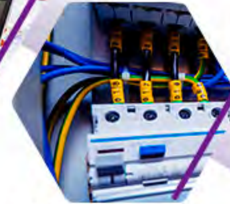
PANELES DE CONTROL
